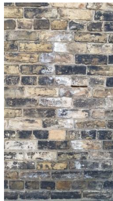
Figure 35: Efflorescence of the bricks.
