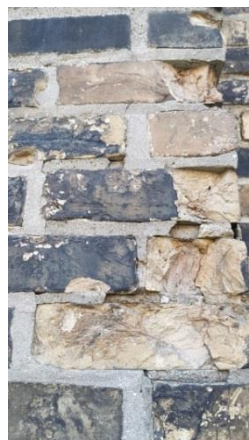
Figure 20: Loss of face of bricks.
