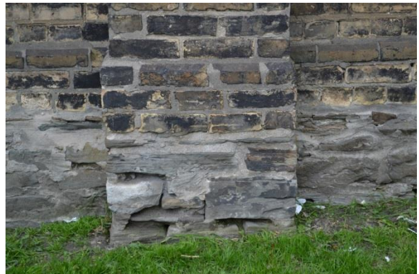
Figure 40: Erosion and surface loss of foundation stones.
