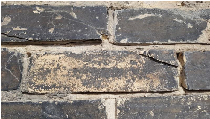
Figure 23: Close-up of a cracked brick.
