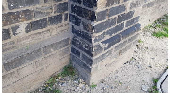
Figure 22: Missing ledge of plinth course with mortar patch.
