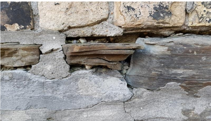
Figure 38: Splitting of stone along shale planes.
