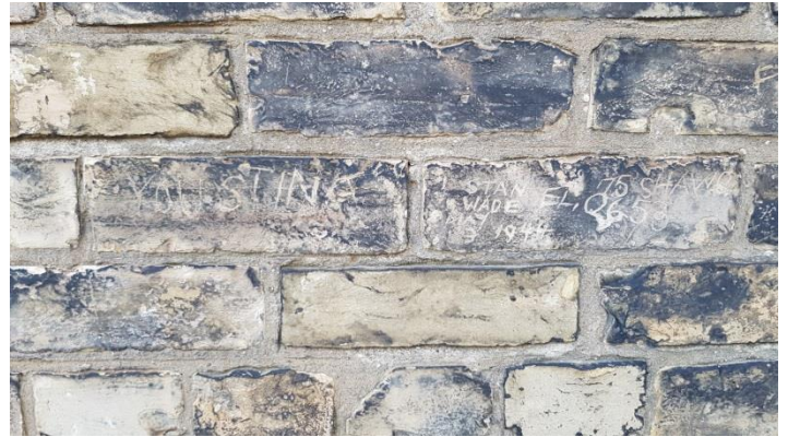
Figure 33: Scratch graffiti on the surface of the bricks.
