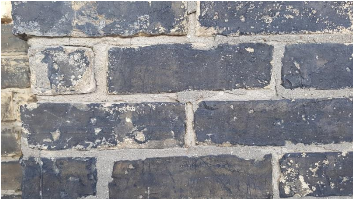
Figure 28: General atmospheric soiling on bricks.
