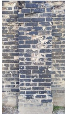
Figure 29: General atmospheric soiling on bricks.
