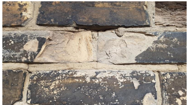
Figure 18: Example of surface loss due to erosion.
