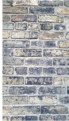
Figure 27: Small gouges from ivy left in surface of bricks.
