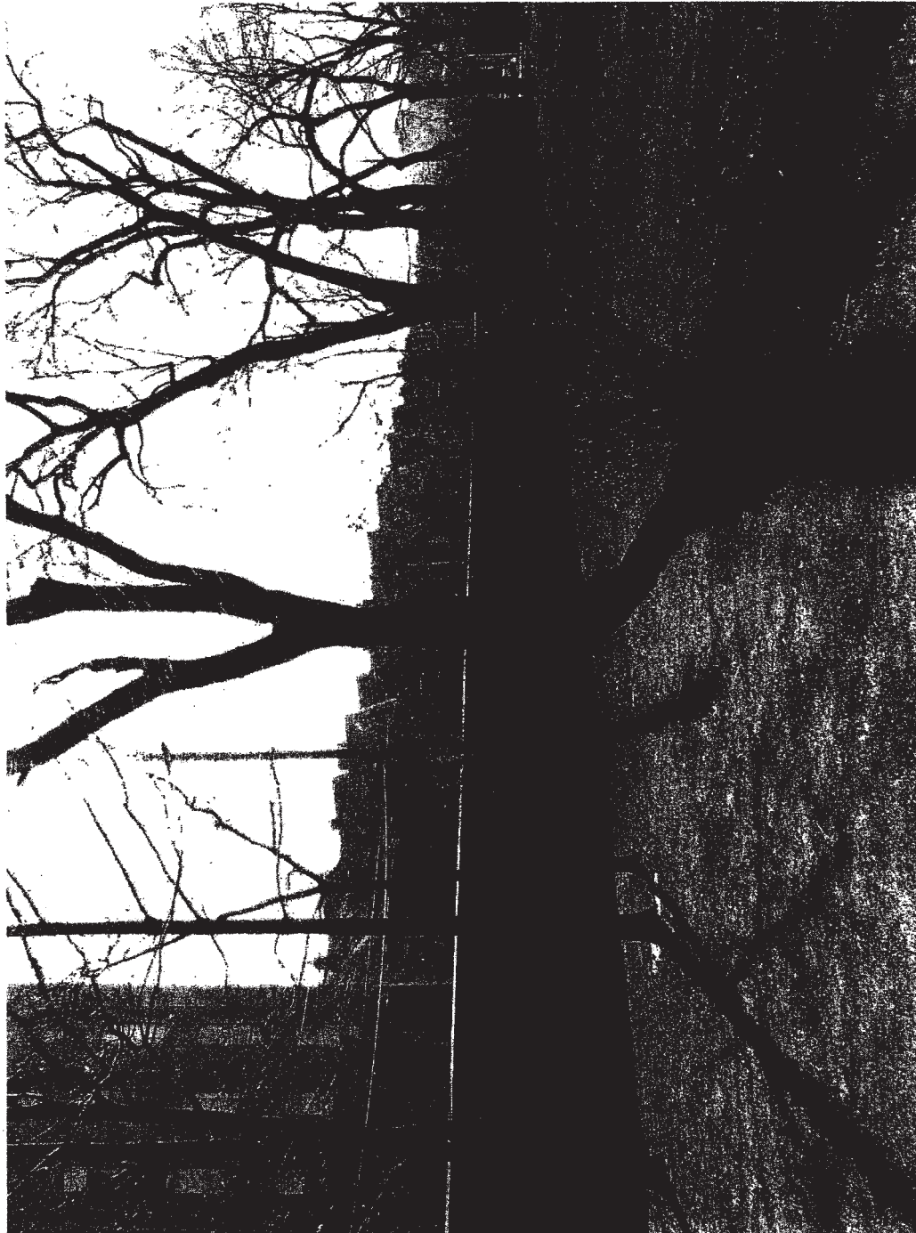
View of the east section of the wall, showing the west face with the change in height and, toward the south end, one of the two oversized openings in the wall.
