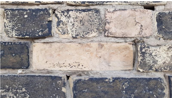
Figure 17: Example of an eroded brick.
