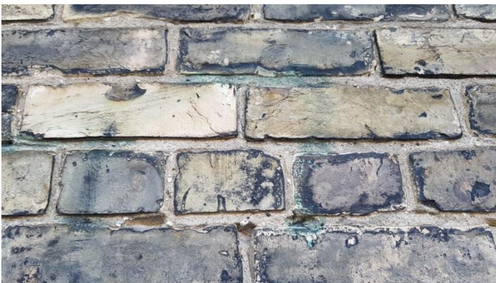
Figure 36: Traces of copper staining on the bricks and mortar.
