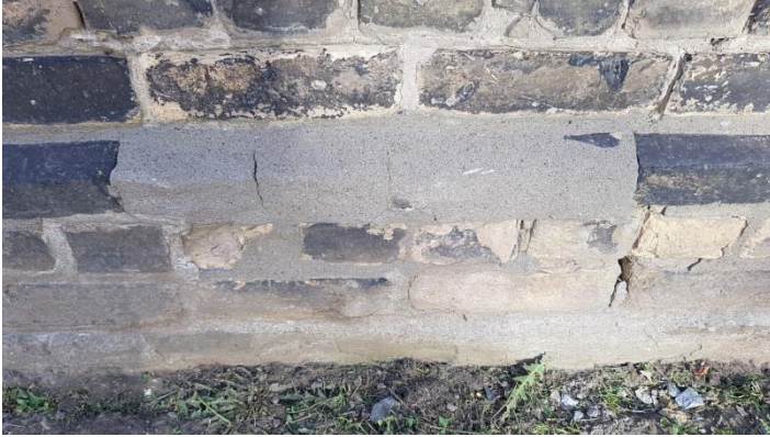
Figure 21: Missing ledge of plinth course with mortar patch.
