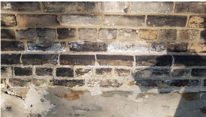
Figure 34: Efflorescence of the bricks.
