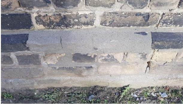
Figure 45: Damaged plinth course to be replaced with salvaged bricks.
