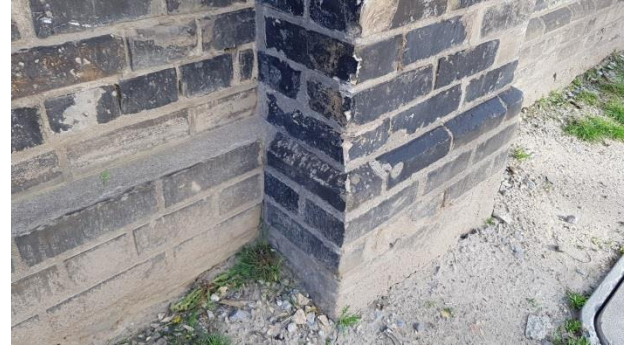
Figure 46: Damaged plinth course to be replaced with salvaged bricks.
