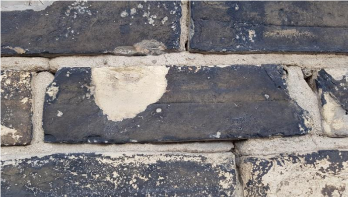
Figure 16: Example of a spalled brick.
