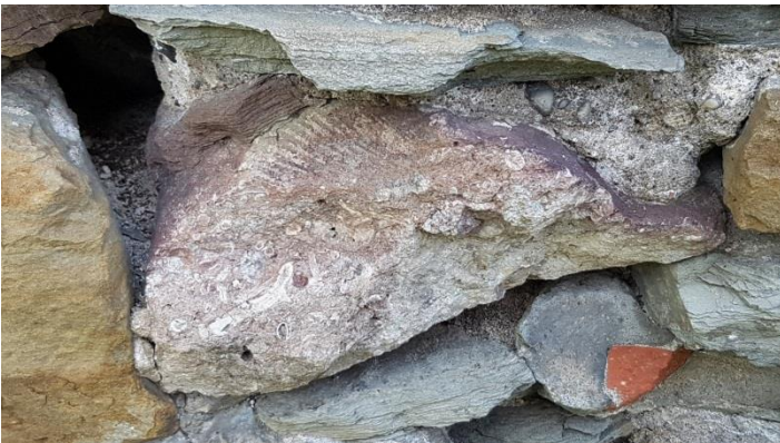
Figure 39: Erosion and surface loss of foundation stones.
