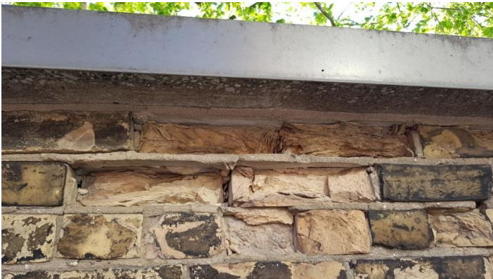
Figure 24: Hard mortar causing deterioration of bricks.
