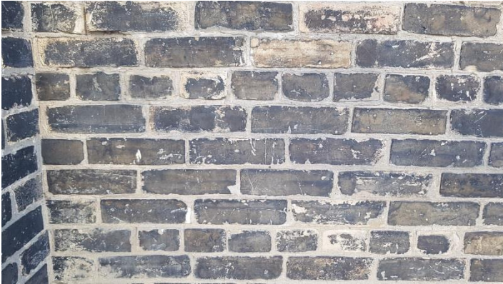
Figure 26: Small gouges from ivy left in surface of bricks.
