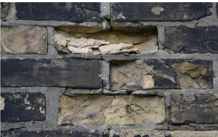
Figure 19: Loss of face of bricks.
