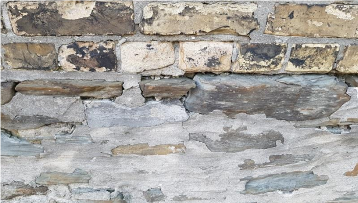
Figure 37: Deterioration of stone foundations along bedding planes.
